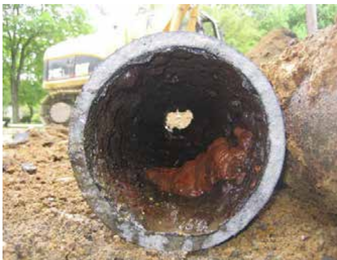
Tuberculation of water main
